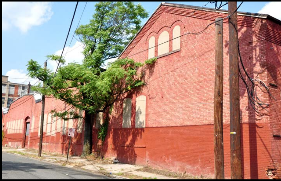
NATIONAL 1: Oblique overview of Dye Houses and Boiler House (right) looking northwest along Piercy St. from corner of Presidential and Piercy.
