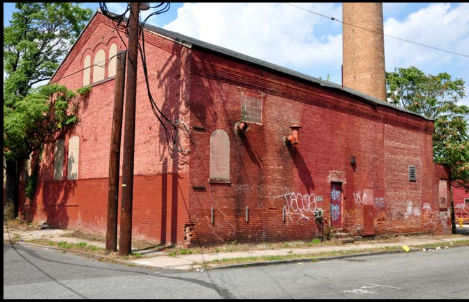
NATIONAL 5: Oblique view of the Boiler House looking north from the corner of Piercy St. and Presidential Ave.
