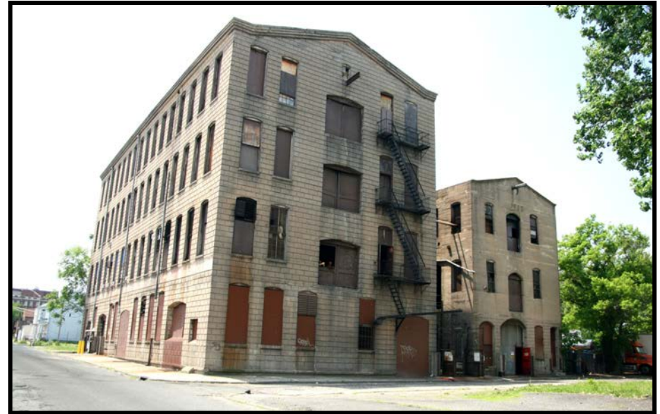
SOWERBUTT 2: oblique overview of north gable ends of both mills, looking southwest from across Paterson St. toward corner of Harrison and Paterson St.
