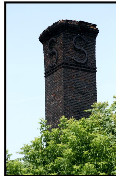
SOWERBUTT 8: Detail view of top of the square smokestack, looking northwest. Note the "S" iron detail attached, representing Sowerbutt ownership.
