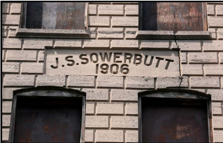
SOWERBUTT 7: Detail view of cast concrete name panel between the third and fourth stories of the east side indicating "J.S. Sowerbutt 1906" ownership and construction date.
