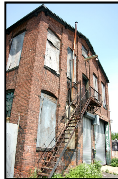
FAIRHURST 2: oblique view of the Fairhurst Silk Mill, previously associated with the Savoy Shirt Co. complex.
