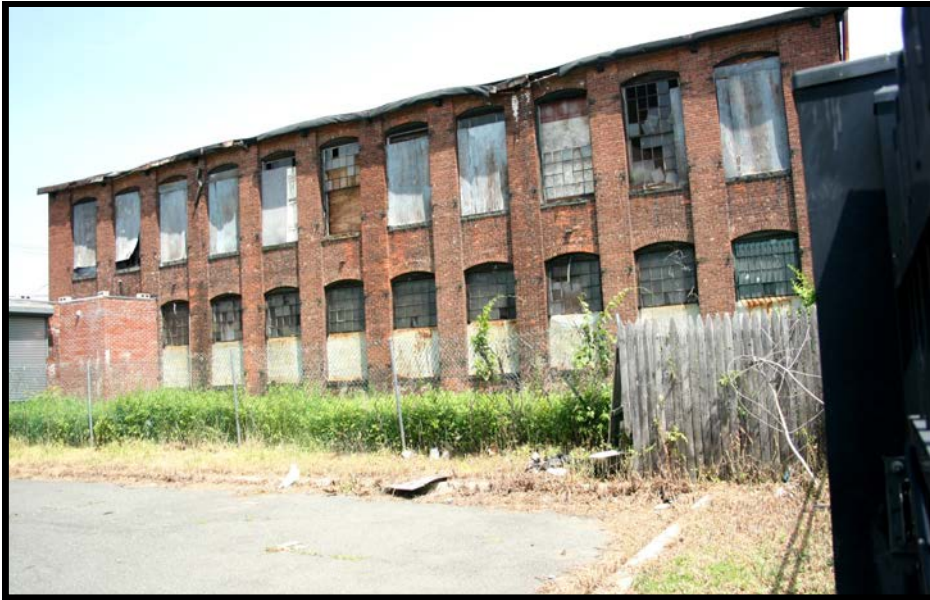
FAIRHURST 3: Oblique overview of the south side of the silk mill, looking north from the adjacent lot along East 18th St.
