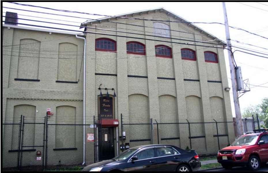
SAVOY 5: View of west side gable end of the south building, looking southeast from across east 18th St.
