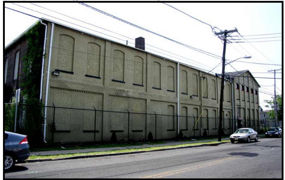
SAVOY 4: oblique overview of north and west sides, looking southeast from across east 18th St.
